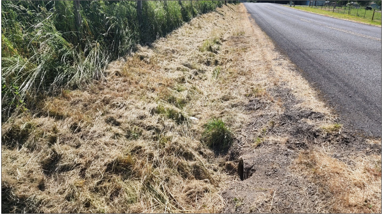
Photo 3. Photo taken from the northeast corner of the site at NE 339 th Street road ditch facing west.
