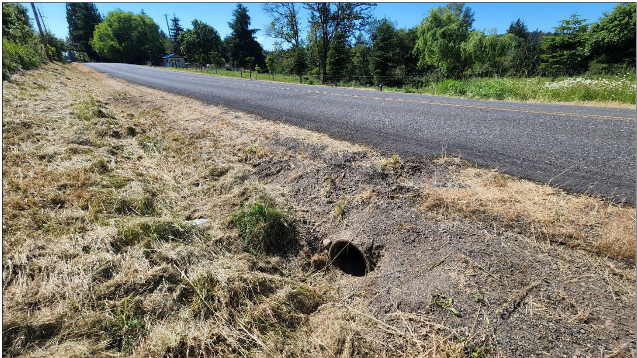
Photo 4. Photo taken from the northeast corner of the site at NE 339 th Street road ditch culvert.
