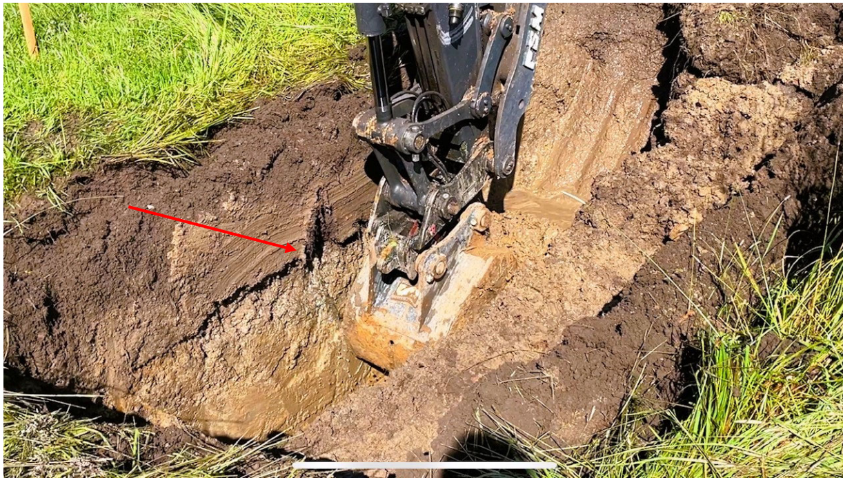
Photo 2. Excavation at TP-5, arrow pointing toward damaged clay drainage pipe; no groundwater observed.
