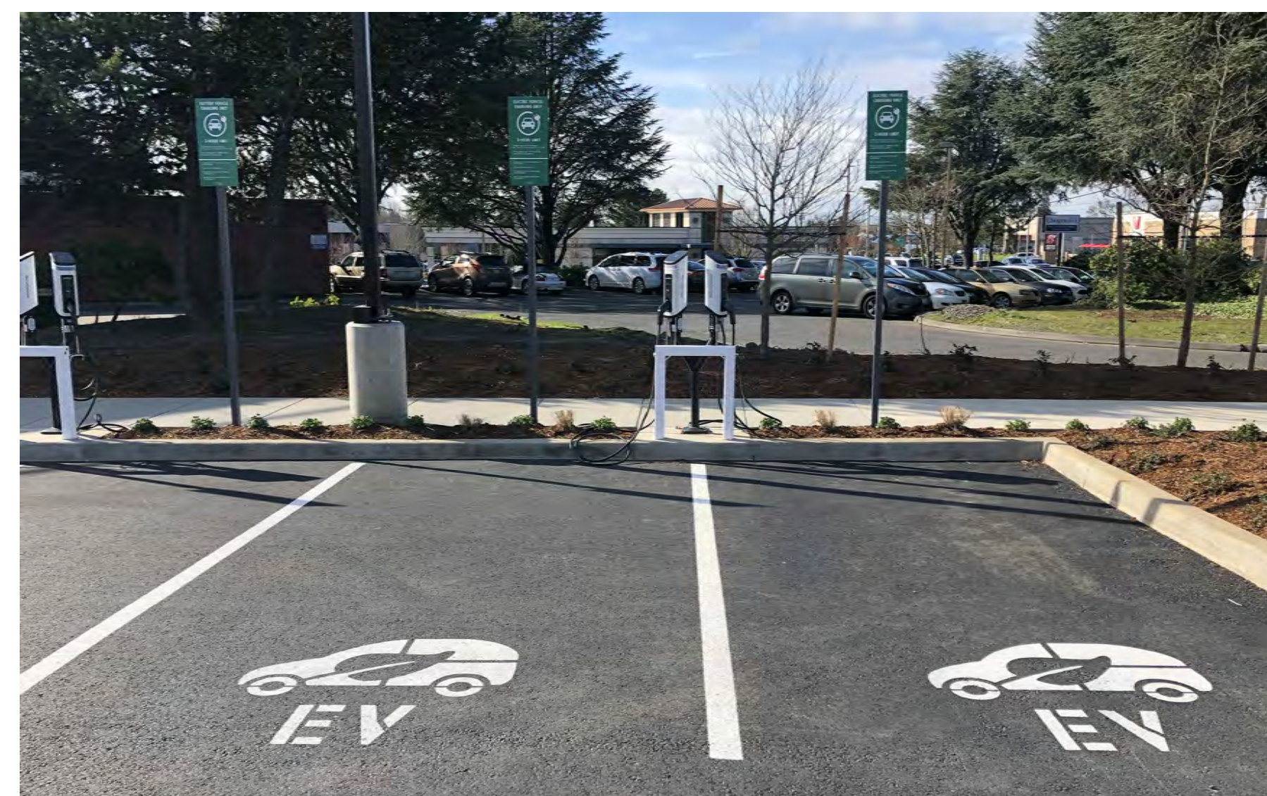
EV CHARGING STATION AT CURB/PARKING SPACE
