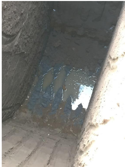
Shallow Groundwater Observed in Several Test Pits
