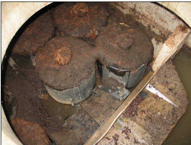
Media Cartridge Filter Vault with Accumulated Sediment
