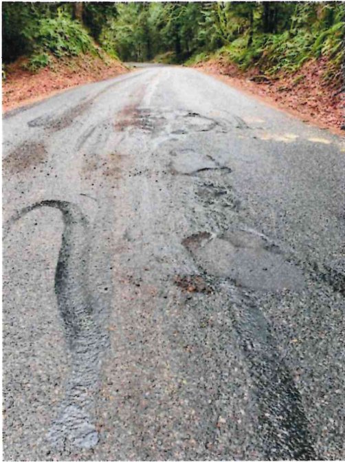
Potholes along Spencer Road looking north
