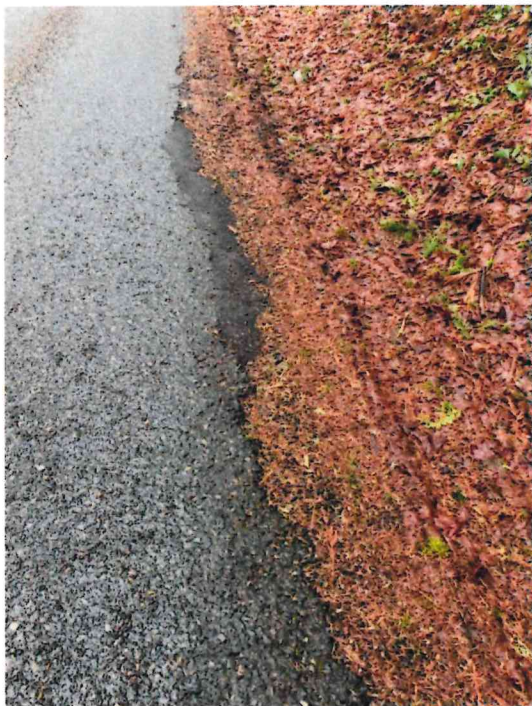
Edge of Spencer Road raveling
