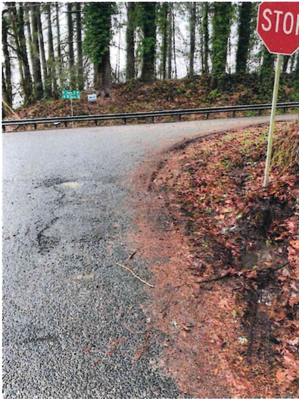
Intersection of Spencer Road and Timmen Road Potholes
