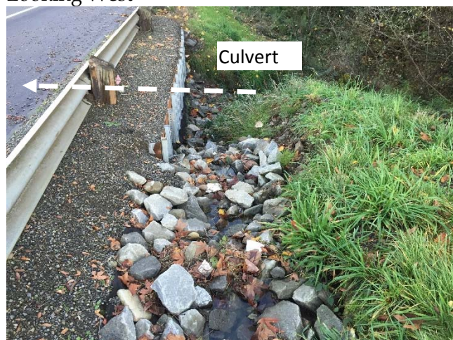
Picture 2.5a: Southside of La Center Rd Looking East above culvert location
