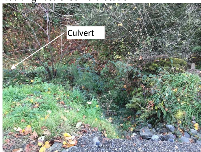
Picture 2.5b: Southside of La Center Rd Looking @ embankment above culvert location
