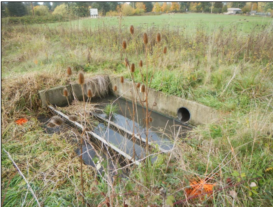
Photo 6. Stormwater control feature. View is to the northwest.
