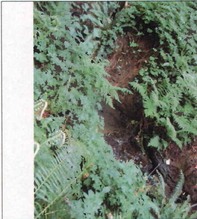
A typical section of the channel in the upstream reaches of the draw. Note the gravel bottom and near-vertical (though stable) slopes. This section is not far below the outfall of the culvert.
