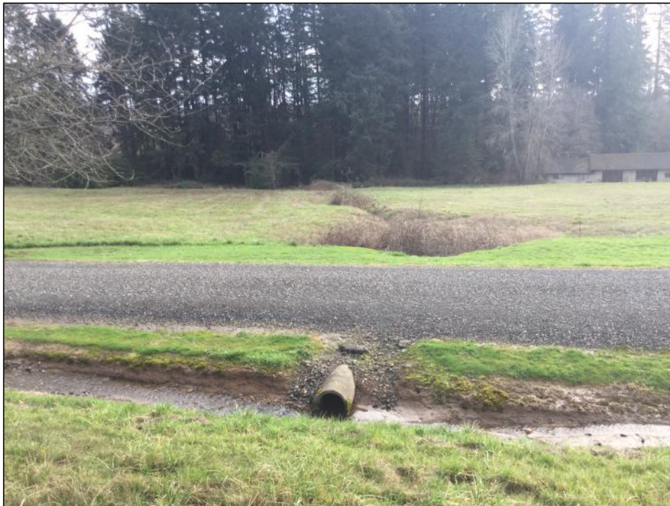
Photo 3 - Drainage ditch along the north side entering culvert to drainage swale/ditch in south pasture of the project area.
