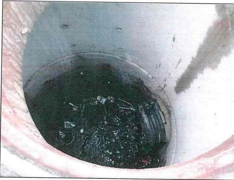
Drywell with Accumulated Trash
