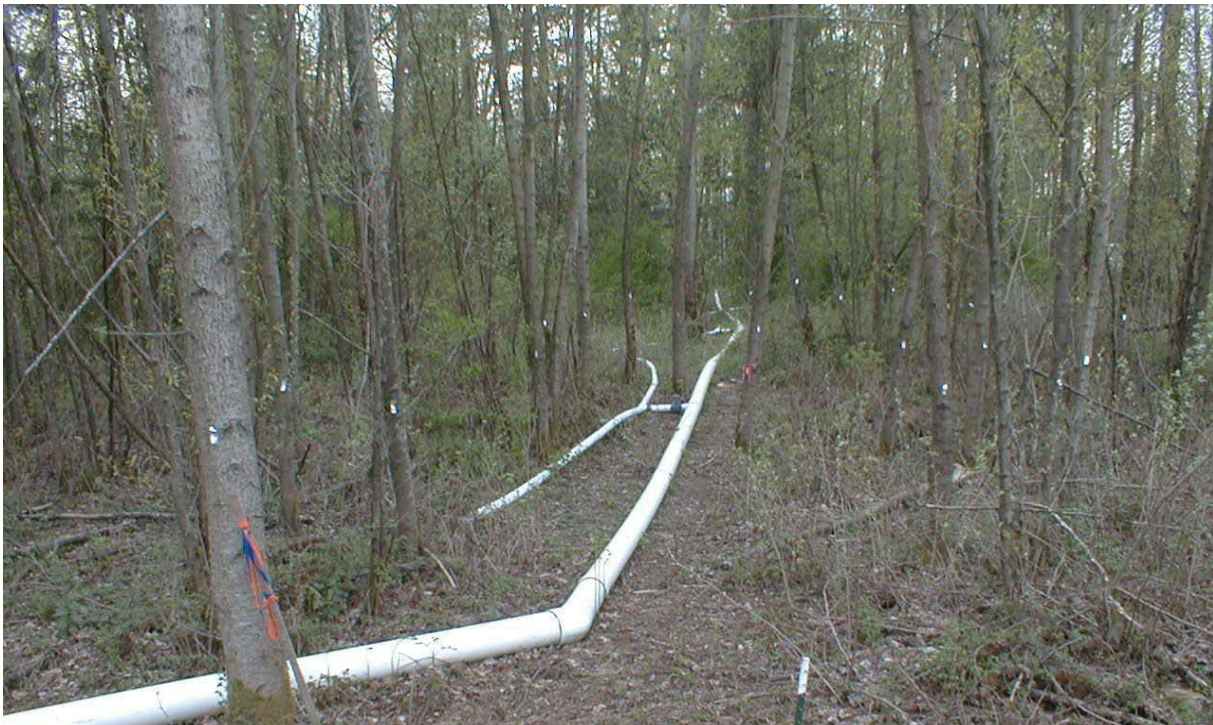
Figure 4.2.15 – Manifold and Braches in a wooded, vegetated spray field
