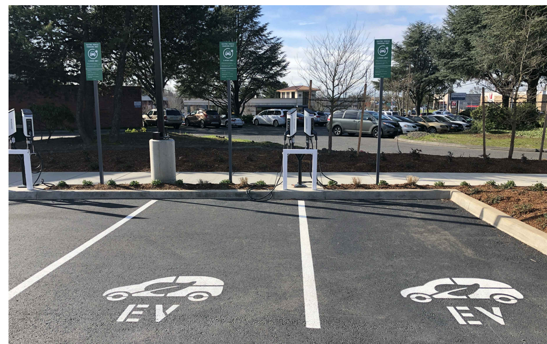
EV CHARGING STATION AT CURB/PARKING SPACE
