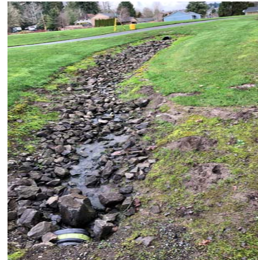
Photo H. View facing northeast of rip-rap lined swale off-site where Water 1 originates. Photo taken by AKS survey crew on 12/02/2018.
