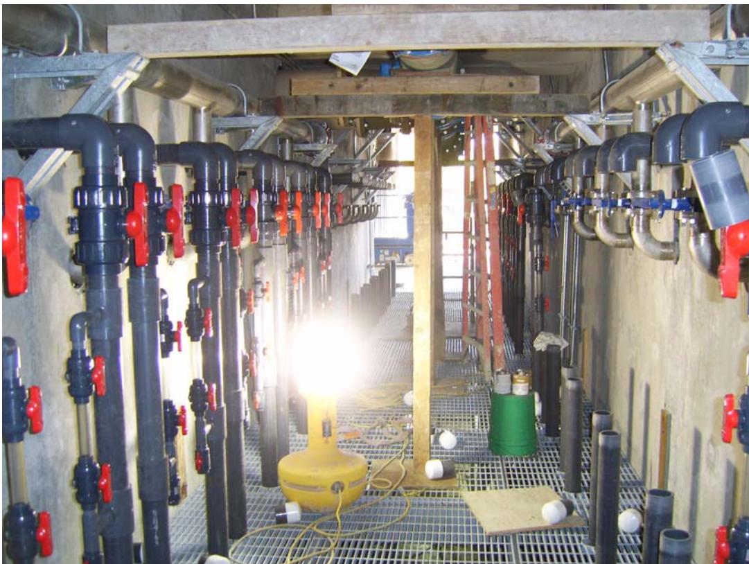
3/26/10 – Pipe Gallery Piping and Valving
