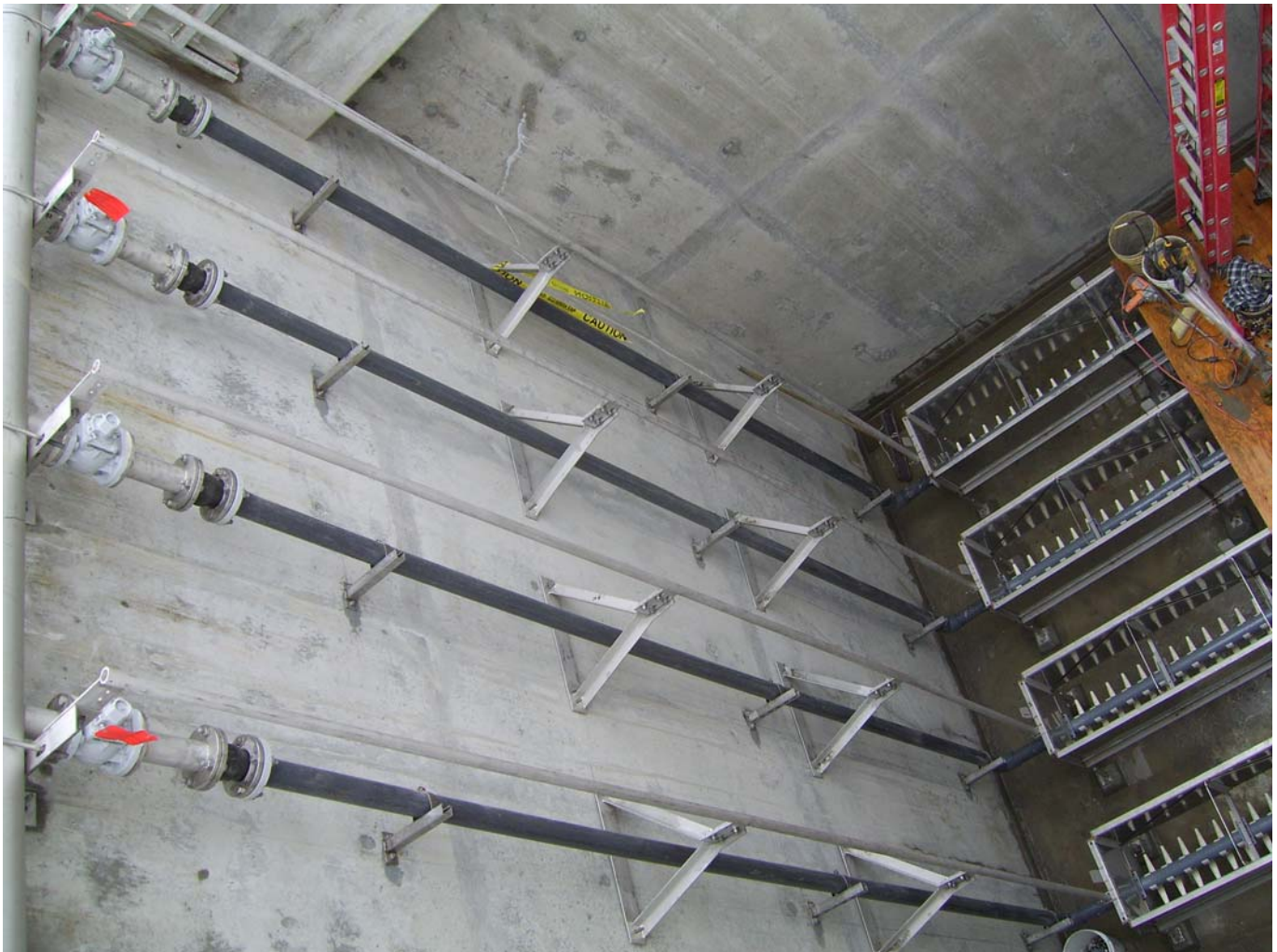
3/25/10 – MBR 2 diffusers and piping
