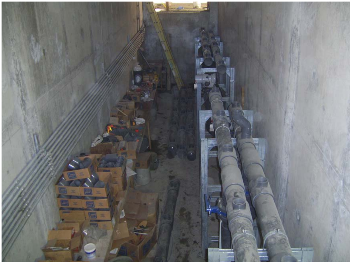
2/18/10 – Piping and Conduits in MBR Pipe Gallery
